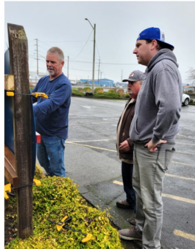
David Anderson, David Cox and Eric Kinnaman make sure it's level before the final install.
